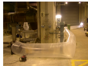
Ducts for removal of styrene fumes when working with thermosetting polymers.
